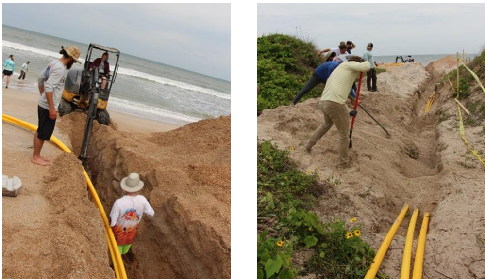
Figure 3 – Left: Excavating the trench across the dry beach and installing the three conduits. Right: Backfilling the trench and burying the conduits.
